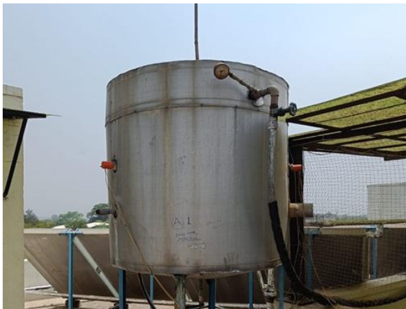
Solar Heaters Installed
