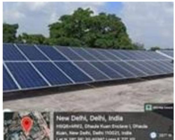
Solar PV Installed
